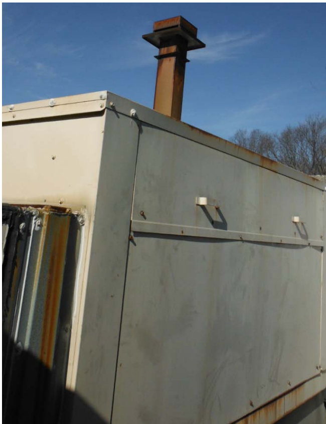
Photo #8: Existing oil-fired unit serving the library addition. Notice the corrosion that is on the unit.
