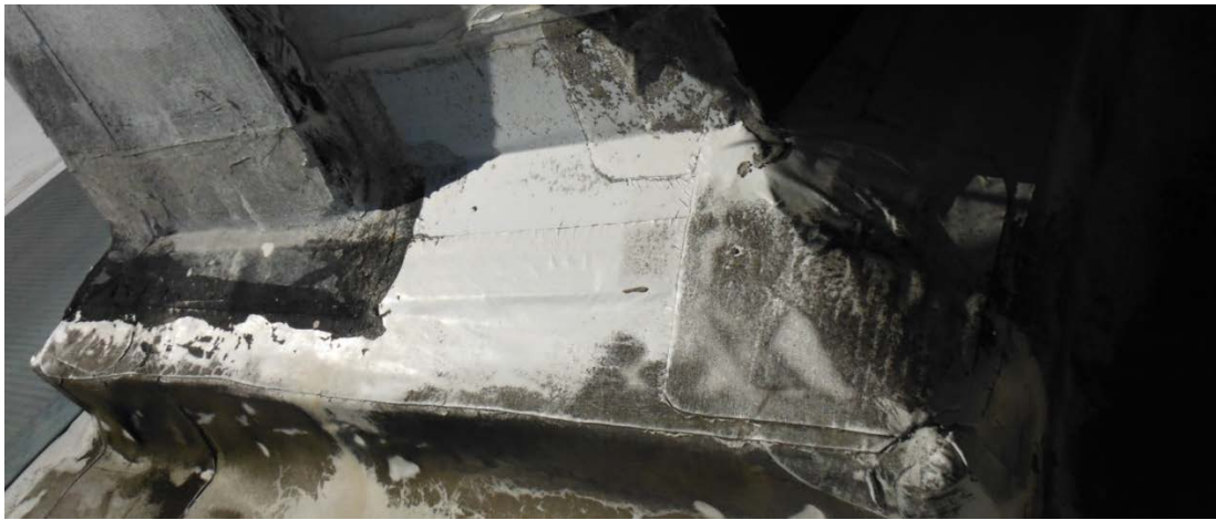
Photo 9: Example of degraded rooftop unit supports.
