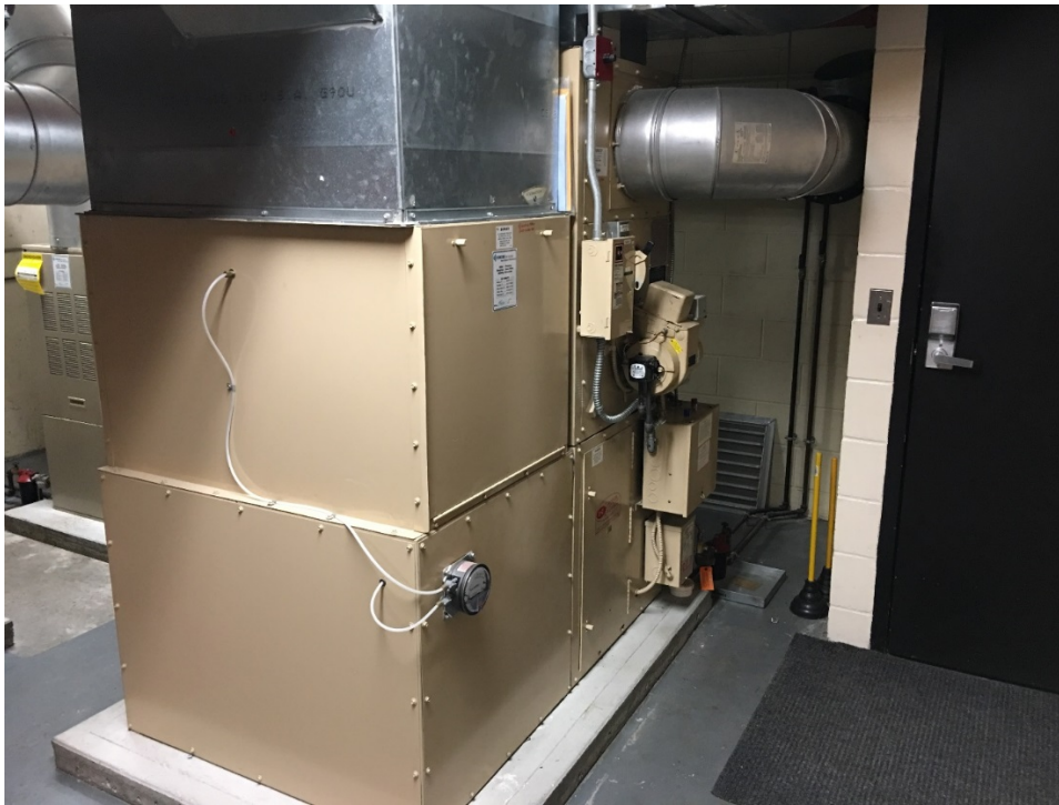
Photo #13: Existing oil-fired heating, non-cooling air handling unit. The unit appears to be in good condition but is closely approaching 20 years of service.
