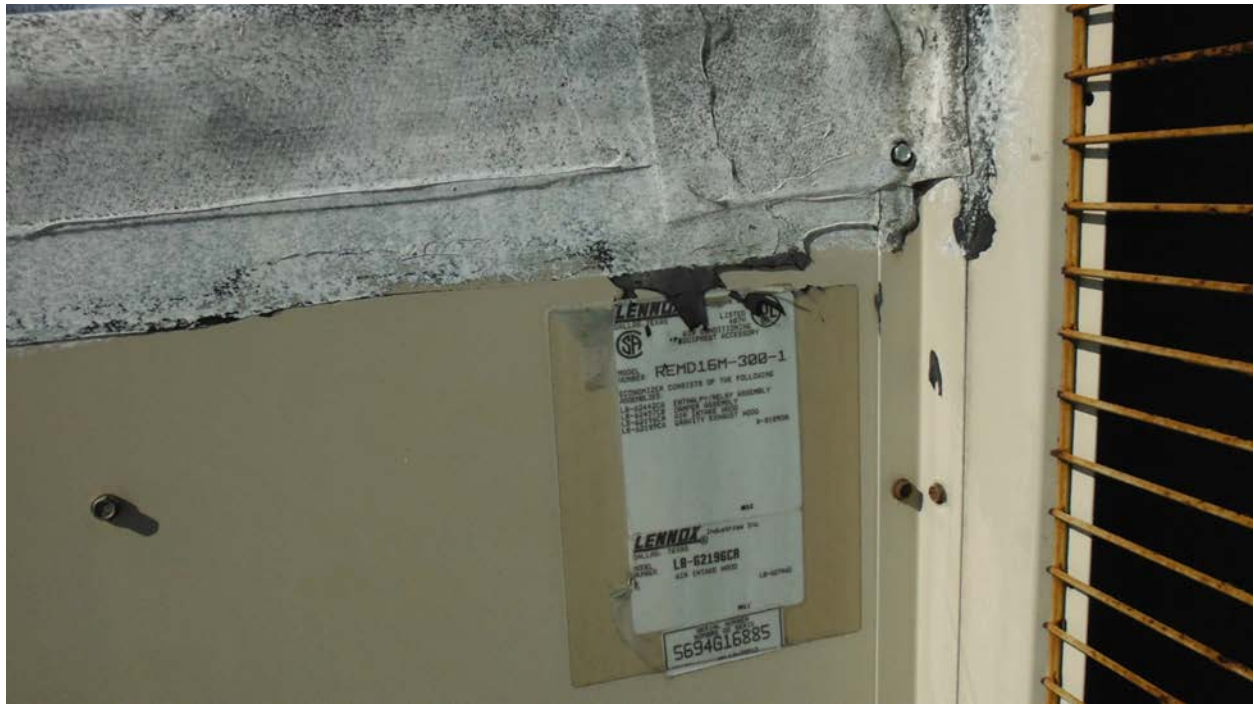
Photo 3: Rooftop cooling only unit with degraded mastic.
