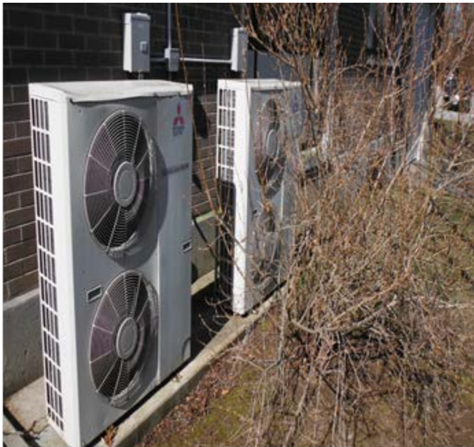
Photo #6: Condensing unit serving the conference room space.
