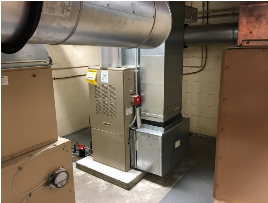
Photo #11: Existing oil-fired heating, non-cooling air handling units located in the basement MER. The units appear to be in good condition but are closely approaching 20 years of service.
