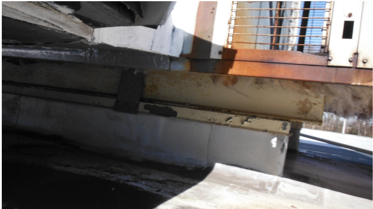
Photo 4: Public Library oil-fired rooftop unit showing the corrosion on the unit itself.
