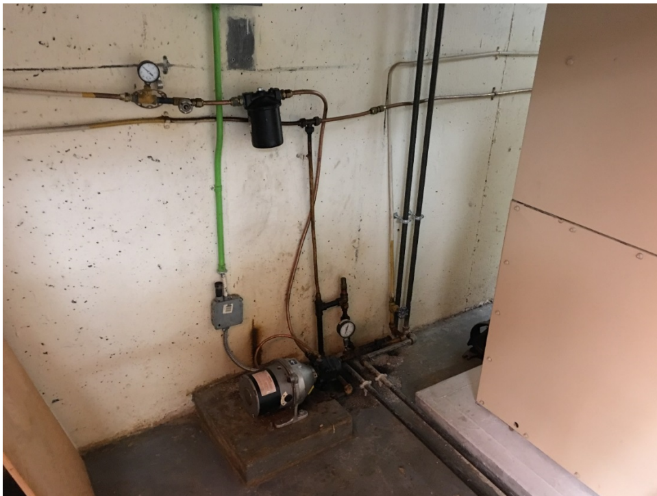
Photo #14: Fuel oil transfer pump. The unit appears to be in good condition but exhibits signs of leaking.
