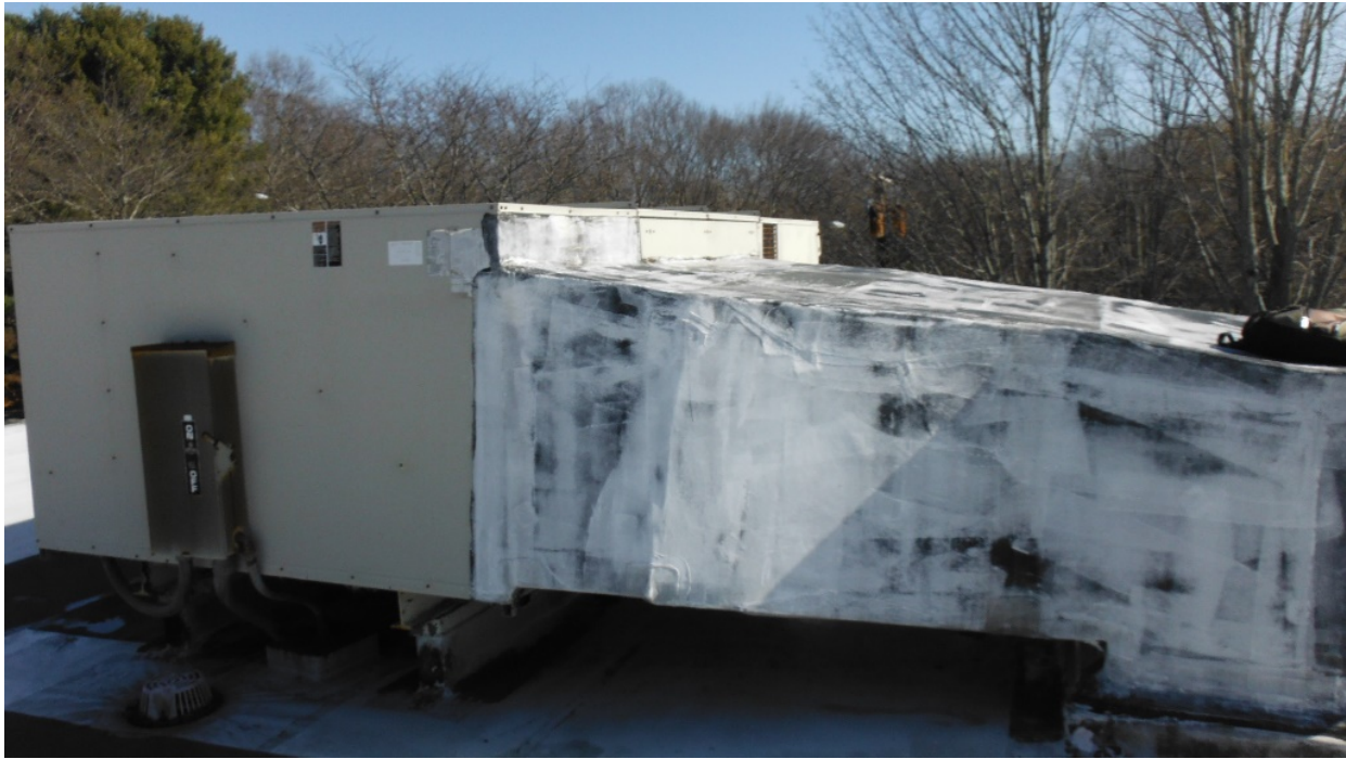
Photo 1: Rooftop cooling only unit. Exterior insulation on the duct work is no longer attached.
