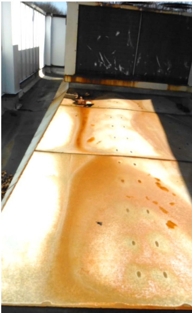
Photo #10: Existing oil-fired unit serving the library addition showing the corroded curb adapter.
