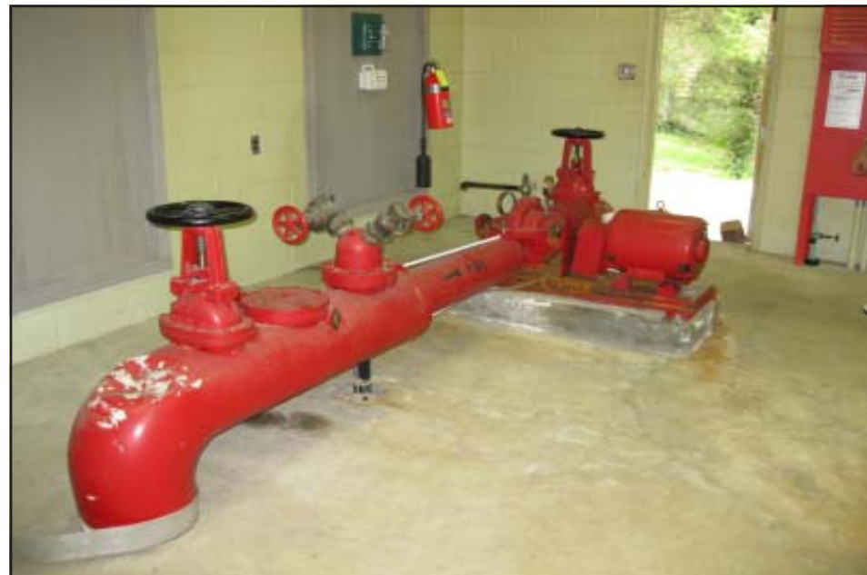
Photo 4 - Fire pump on ground floor level.
