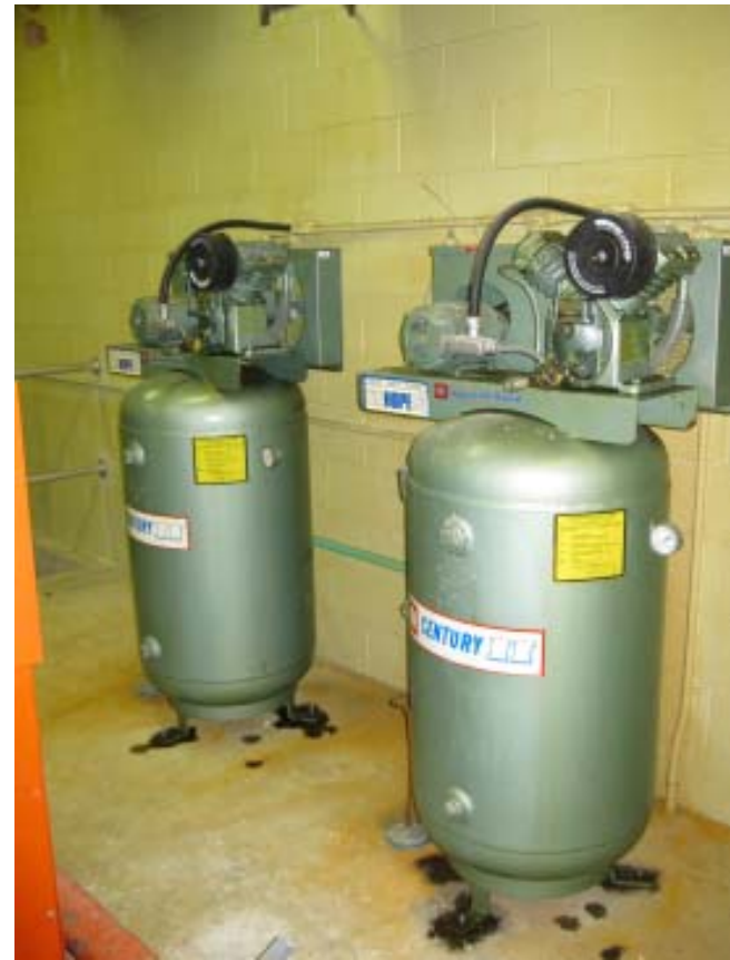
Photo 6 - Air compressors on ground floor level.
