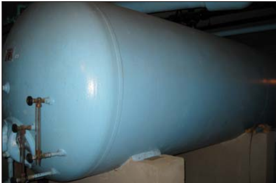
Photo 7 - One of two 2500 gallon pneumatic tanks in basement level.
