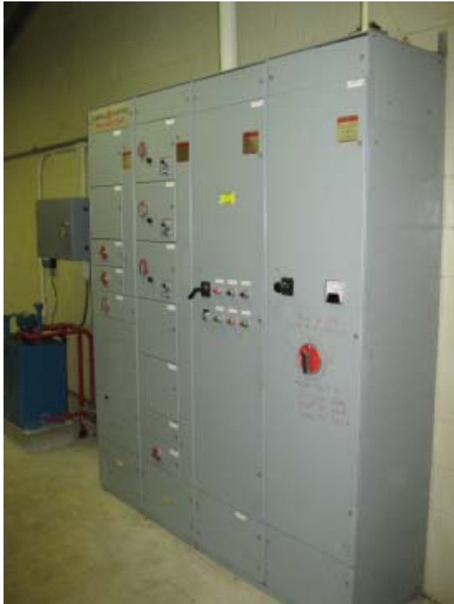
Photo 5 - Motor control center on ground floor level.
