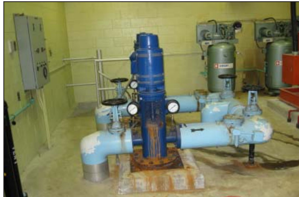
Photo 2 - Domestic pumps on ground floor level.
