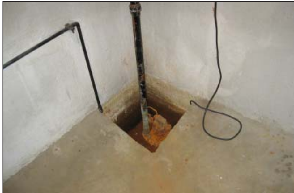
Photo 8 - Existing sump pump in basement level.
