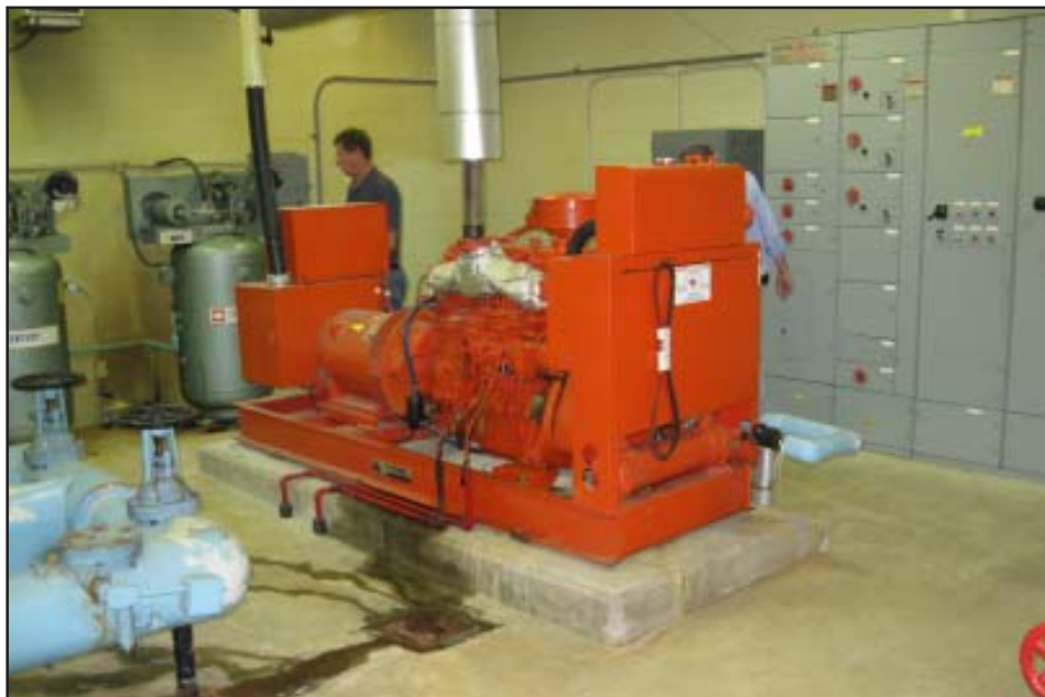
Photo 3 - Diesel engine generator on ground floor level.
