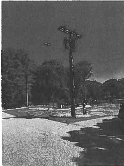
Pole mounted transformer to be replaced with pad mounted ground transformer
