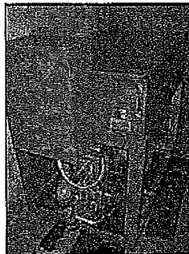
Existing Power Unit
