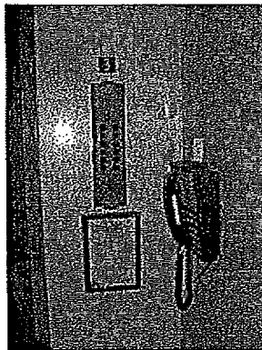
Existing elevator emergency phone
