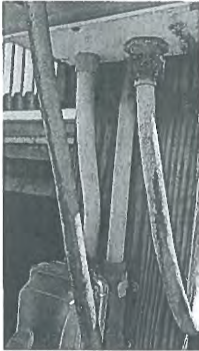
Conduit and connectors showing corrosion
