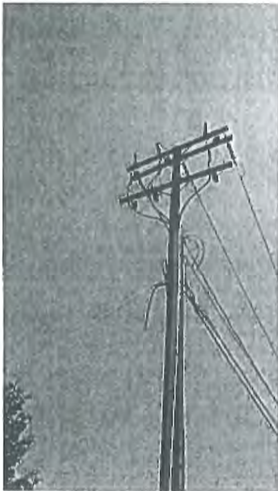
Riser on utility pole for Mago Dock electrical service
