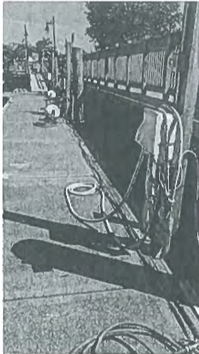
Ship to shore Cable
