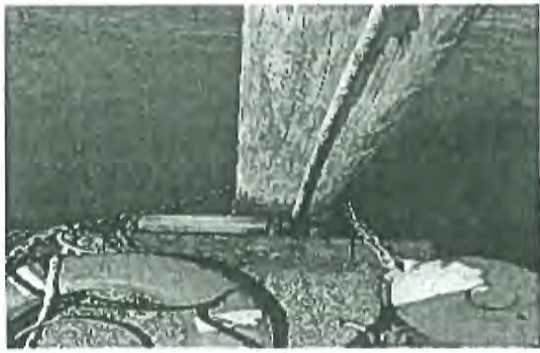
Looking West – Rusting of Finger-Pile Connection
