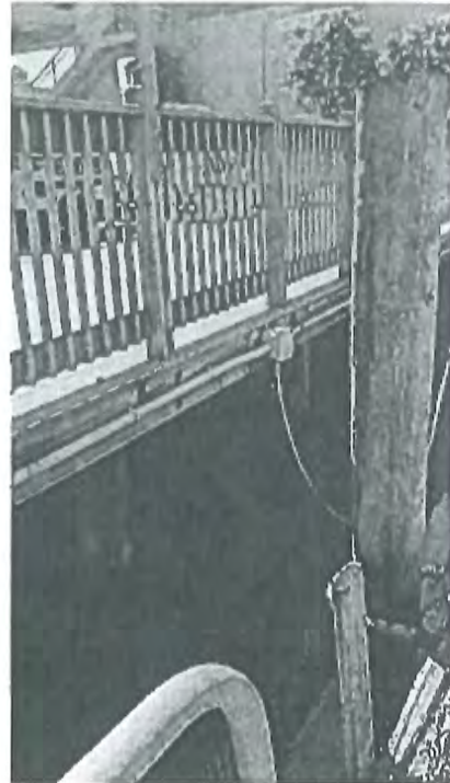
Conduit and junction boxes along rim joist where power pedestals connect to main power.
