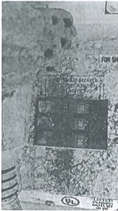
Power pedestal interior
