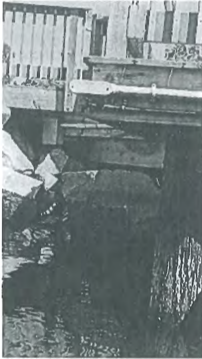
Conduit from junction box (in background) along rim joist to dock
