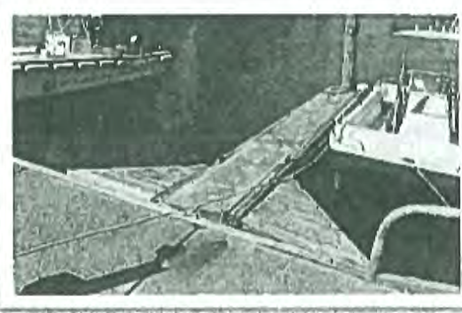
Looking West – First Finger Spalling Concrete & Rust Marks on Precast Concrete Slab
