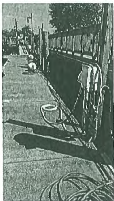
Eaton Newport harbor power pedestals (NP3050)
