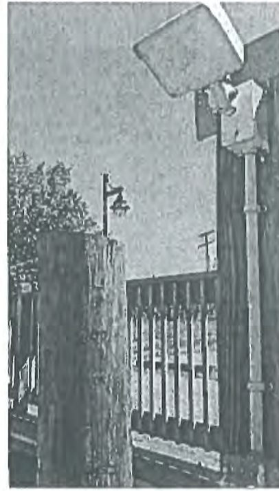
Conduit to light fixture brittle and faded
