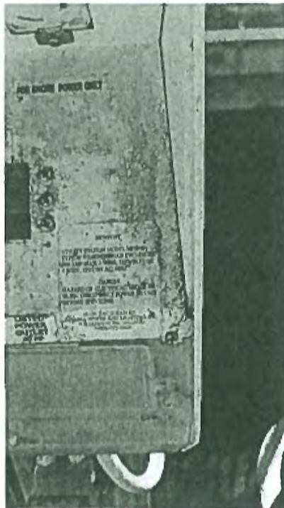
Power pedestal nameplate
