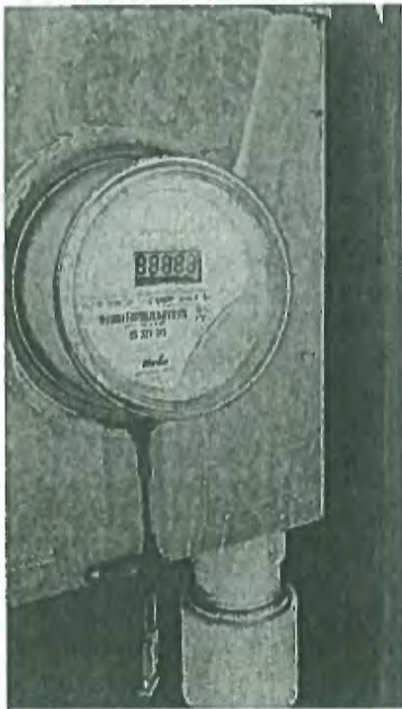
Utility meter for Mago Dock electrical service
