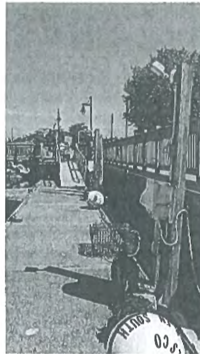
Power pedestal, light fixture and receptacle
