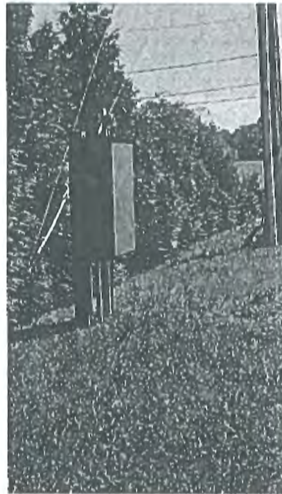
Mago dock electrical service enclosure w/utility pole and riser for the service in background
