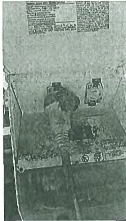
Power pedestal interior
