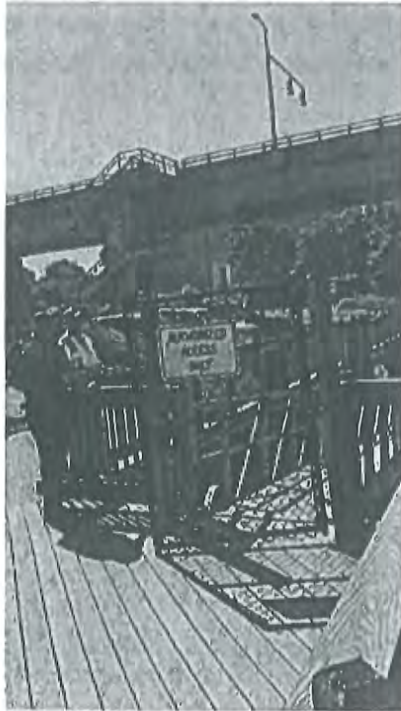
Dock gate with pad lock
