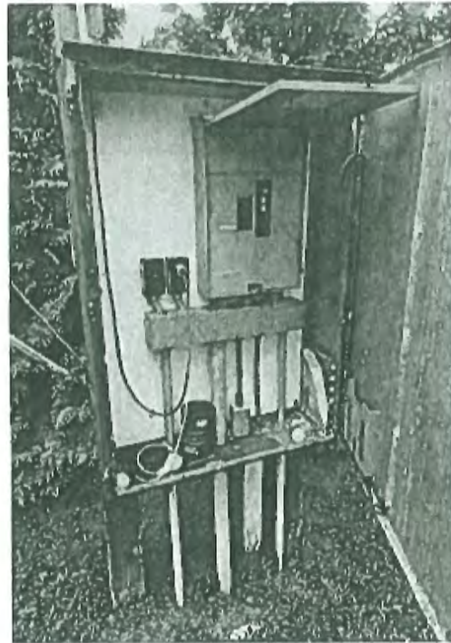
100A panel inside outdoor rated enclosure for Mago dock
