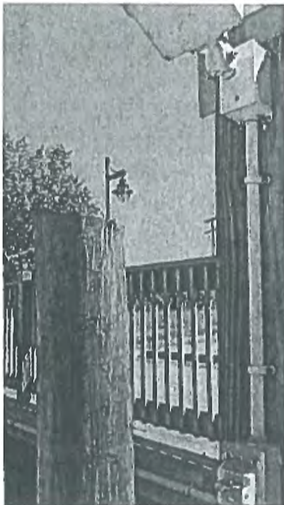
Power pedestal light fixture
