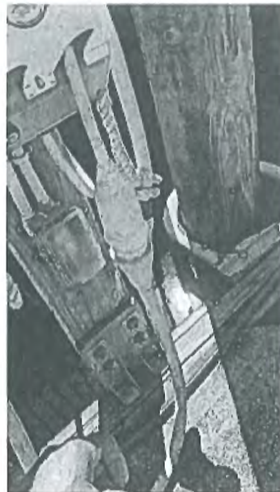
Ship to shore cable with tape on receptacle end.
