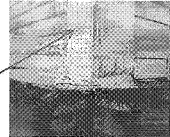
Above – Open Wood Trim Failed Caulk Joint -Peeling Paint
