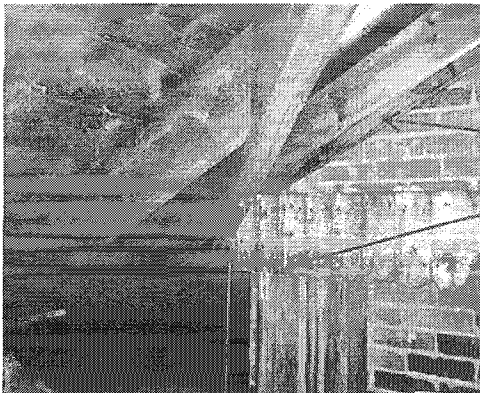
Attic – Interior – Chimney #3 – Western Elevation- Flashing Failure & Masonry Wicking
