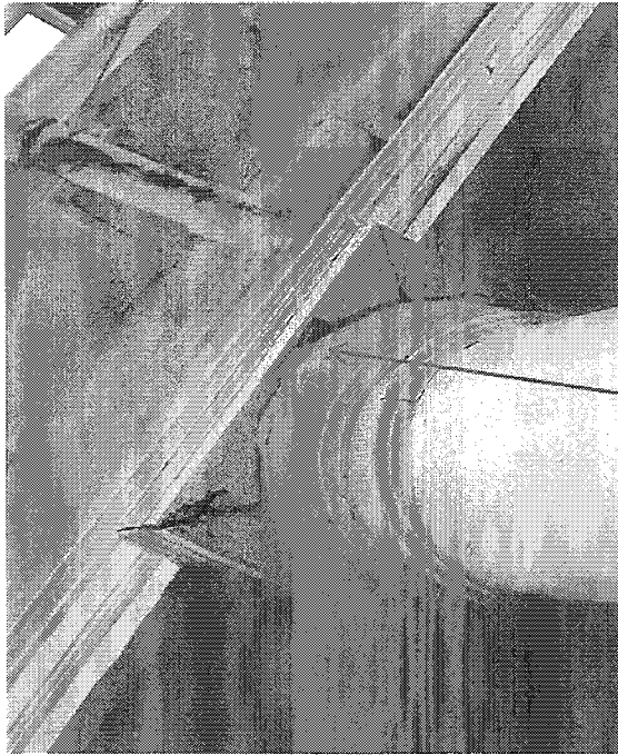
A Leaking Gutter Drain Line is Compromising The Capital of This Doric Porch Column – Along With the Surrounding Trim Work
