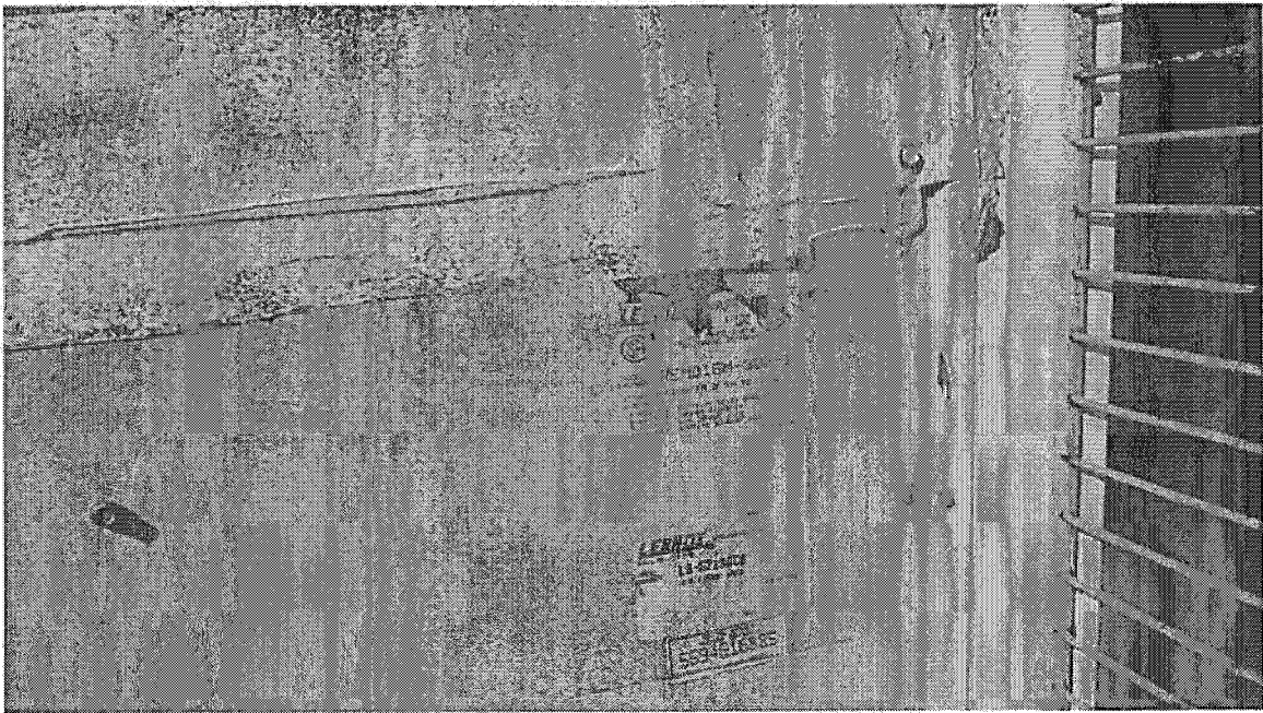
Photo 3: Rooftop cooling only unit with degraded mastic.
