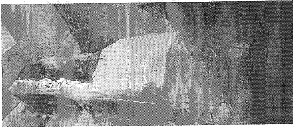
Photo 9: Example of degraded rooftop unit supports.
