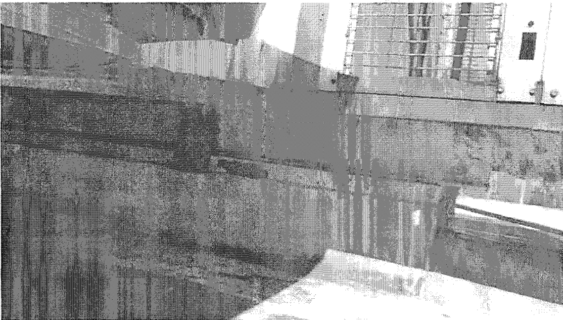
Photo 4: Public Library oil-fired rooftop unit showing the corrosion on the unit itself.
