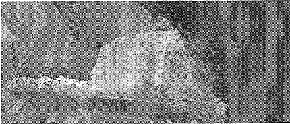
Photo 9: Example of degraded rooftop unit supports.
