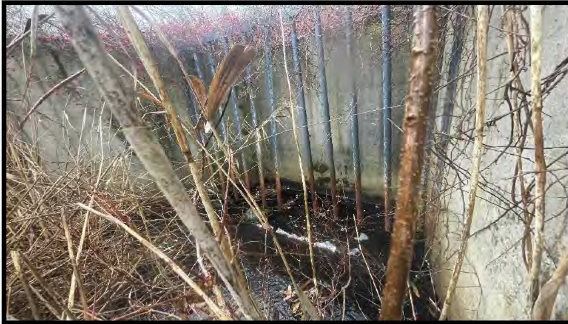
Picture 2 - Detention Basin Outlet Control Structure
