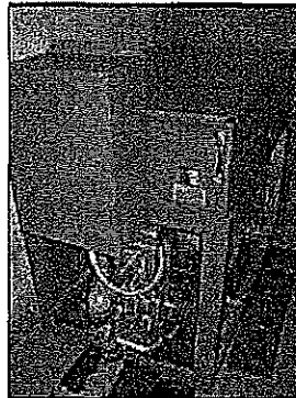
Existing Power Unit
