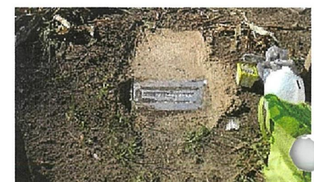
Edge-of-field GKY passive stormwater collector as part of the TLGV RCPP project.
