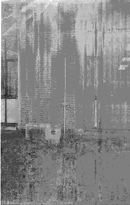
Photo #5: Condensing unit serving the staff office space.
