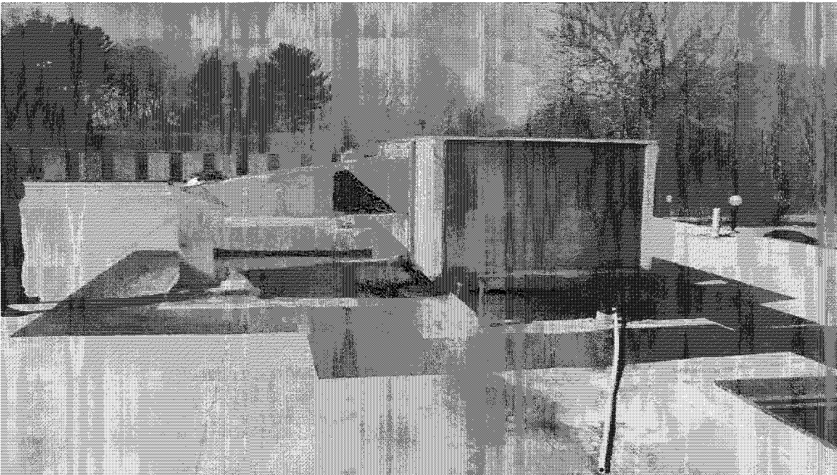
Photo 2: Rooftop cooling only unit. Exterior insulation on the duct work is no longer attached.
