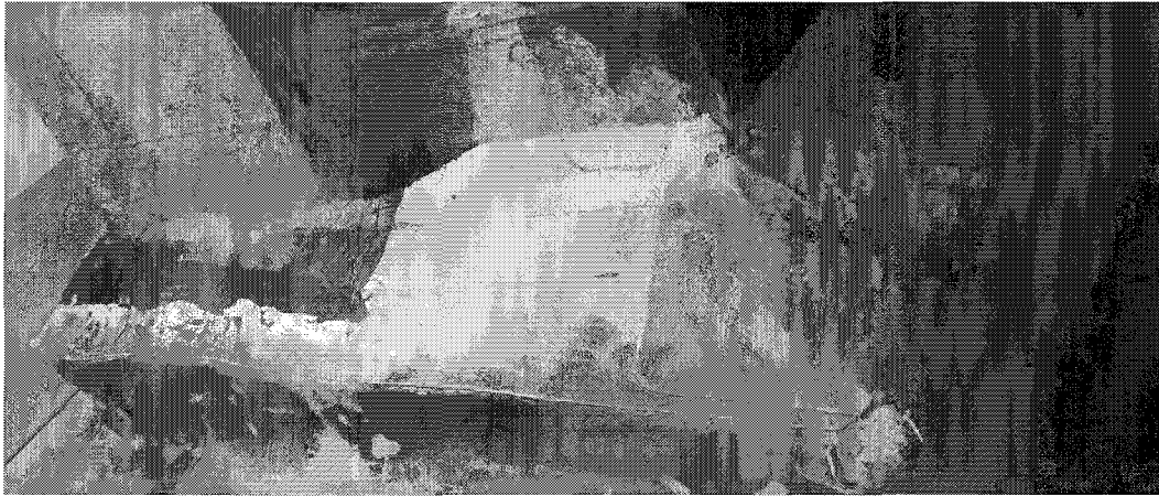
Photo 9: Example of degraded rooftop unit supports.
