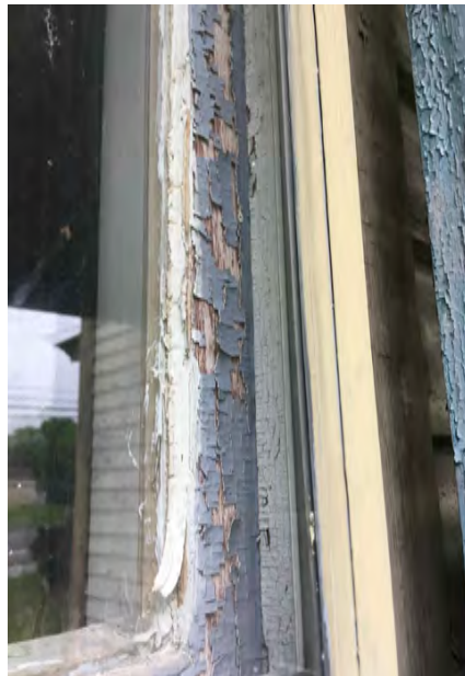
Condition of point on ext'g windows (N) Copper head flashing (typ.)
