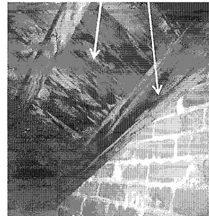
Attic-Chimney #2 Interior Eastern Elevation- Roofers & Framing Previously Saturated
