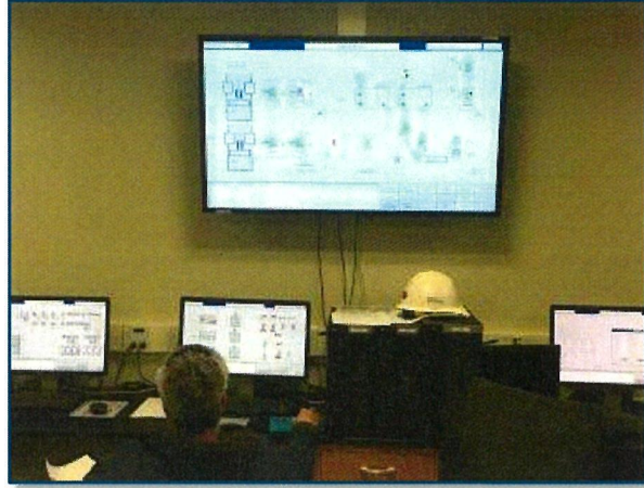
Typical SCADA System Server/Central Station
