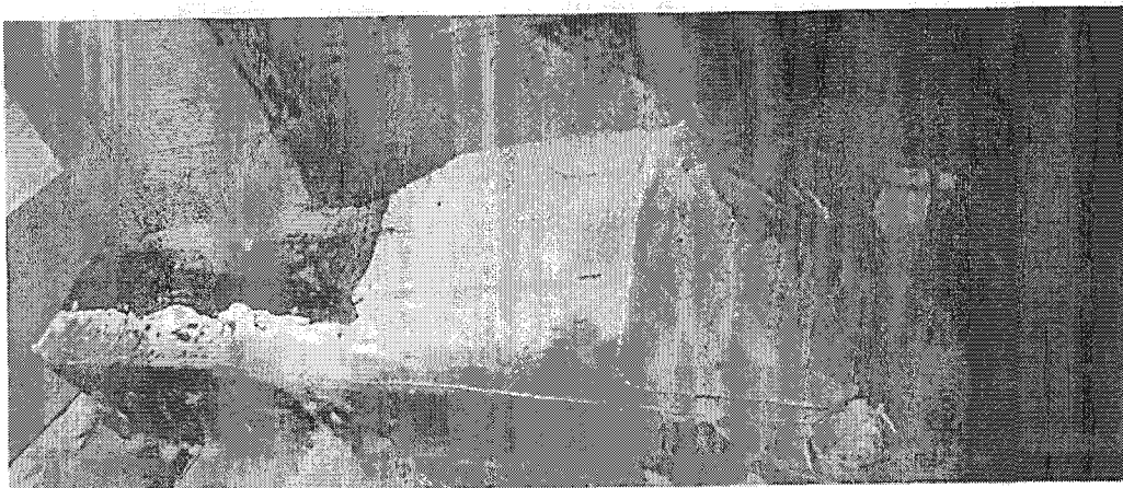
Photo 9: Example of degraded rooftop unit supports.
