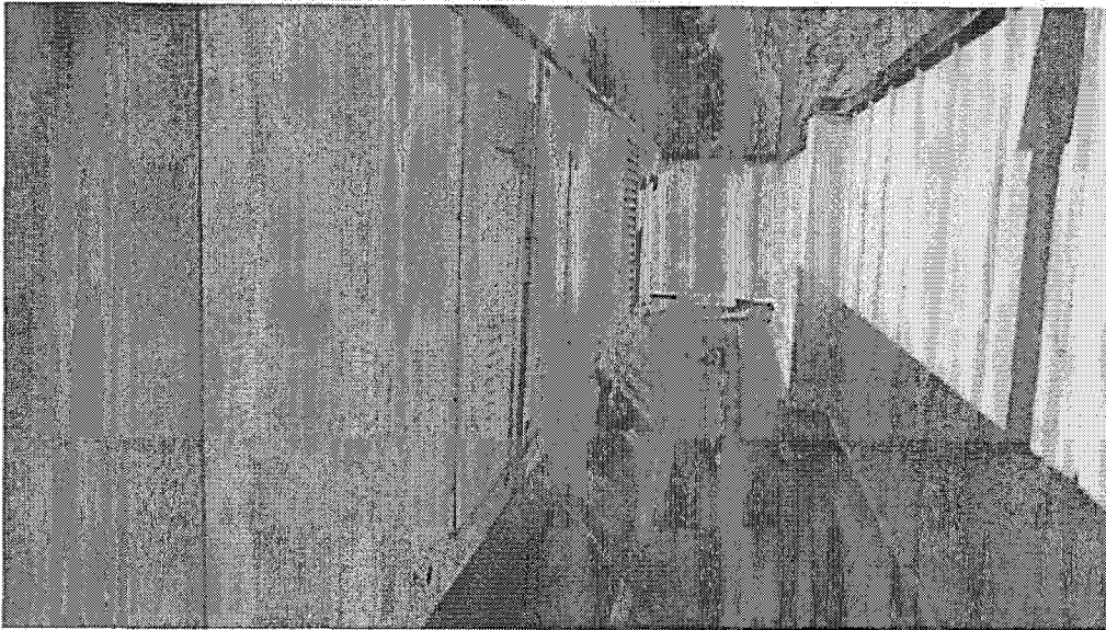
Photo #7: Existing oil-fired unit serving the library addition. Notice the corrosion that is on the unit.
