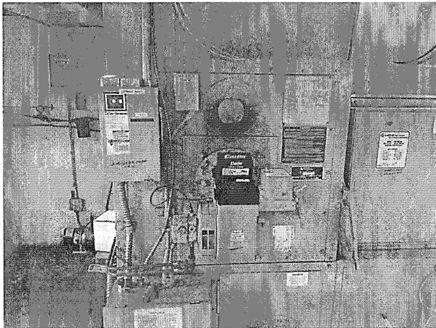
Photo #12: Existing oil-fired heating, non-cooling air handling unit. The unit appears to be in good condition but is closely approaching 20 years of service.
