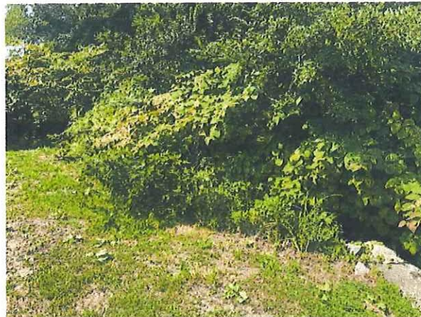
Example of the overgrowth covering the channel on 19 Nichols Lane
