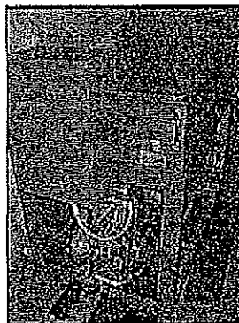
Existing Power Unit
