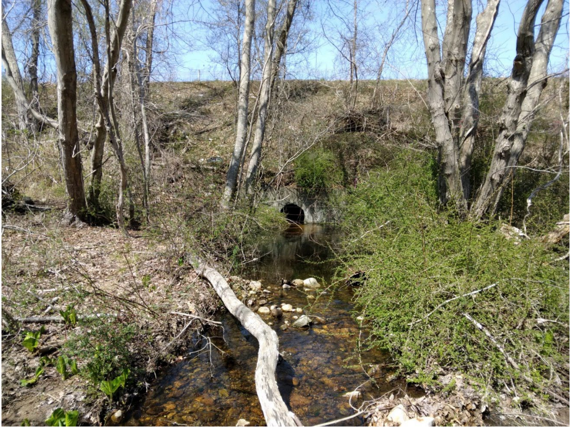
Photograph1 – Wetland 1. Culvert that carries perennial stream under I-95, looking upstream. Note the cobbles and stones collected in the channel, presumably from previous extreme floods as the channel itself does not show erosion. The channel here is 6-8 inches deep and 10-12 feet wide.
