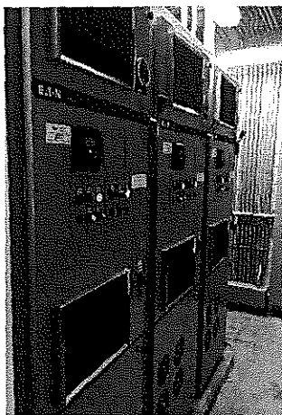
Gurleyville Road Pump Station
