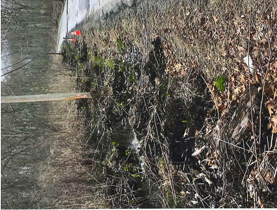
Road east north of failed culvert
