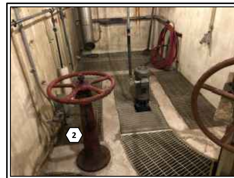
PHOTO WET WELL VALVE 8 -
